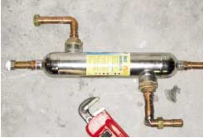
The liberal use of threaded unions allows for easy removal of components for repair or replacement.
