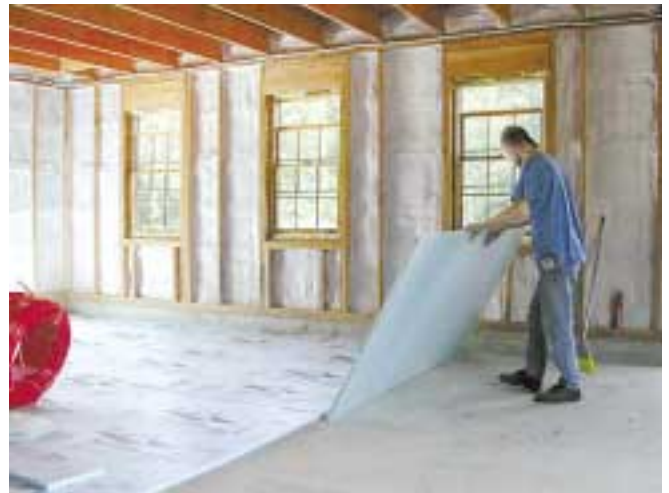
Laying 1 inch polystyrene insulation board over the old floor insulates the heated slab from the earth.
