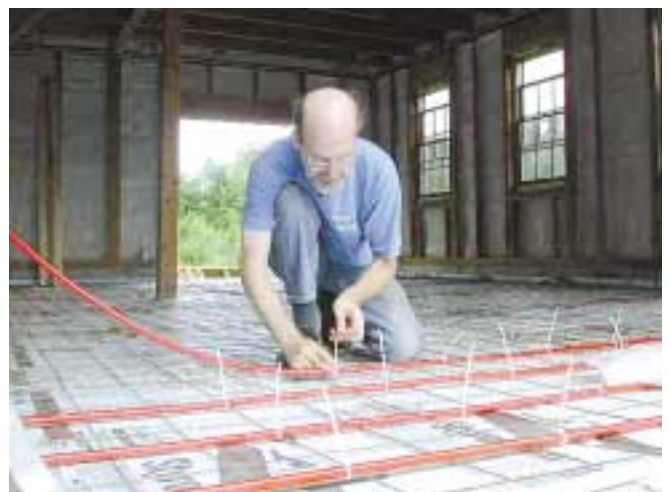
The 600 feet of hydronic tubing is held in place by road wire. Three inches of concrete will make the final layer.
