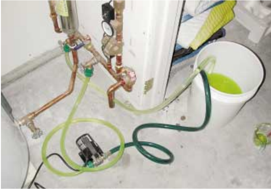
That's not Gatorade! Filling and pressurizing the solar collector loop with the propylene glycol solution.
